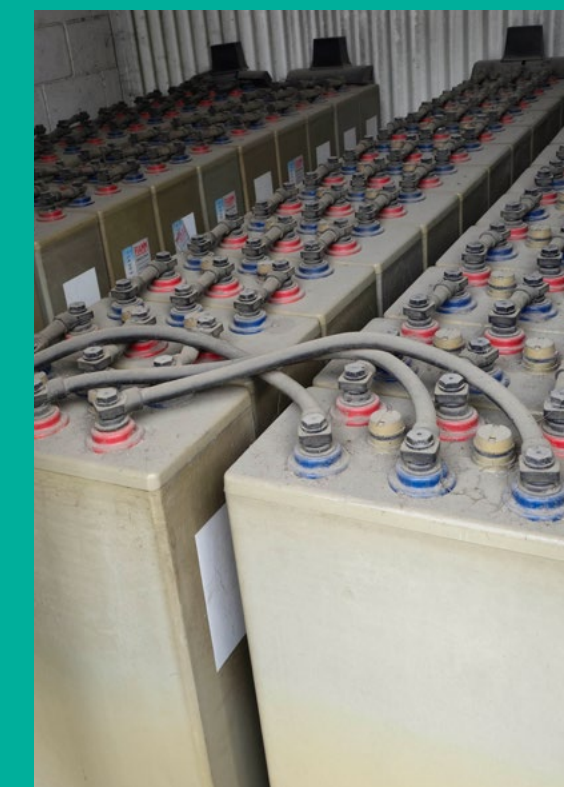
Solomon Islands: Battery system at the Regional Eye Centre, Honiara. 48 × 2V 2500Ah batteries, 240 kWh total capacity.
